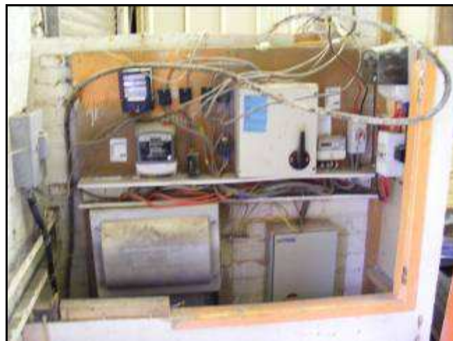
Figure 43 – Existing electrical installation in canoe manufacturer's workshop.
