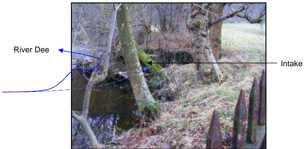
Figure 8 – Dee Valley Water screen and intake.
