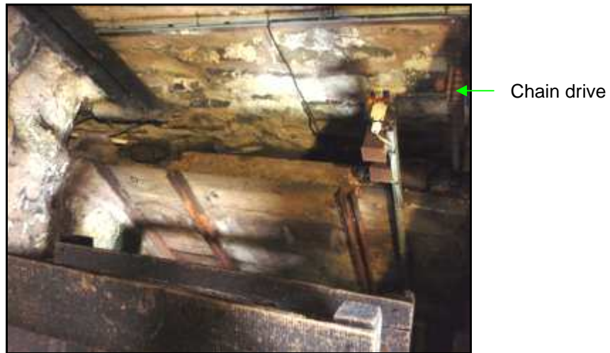
Figure 15 – Corn Mill main sluice gate, control and part of wheel (bottom left).
