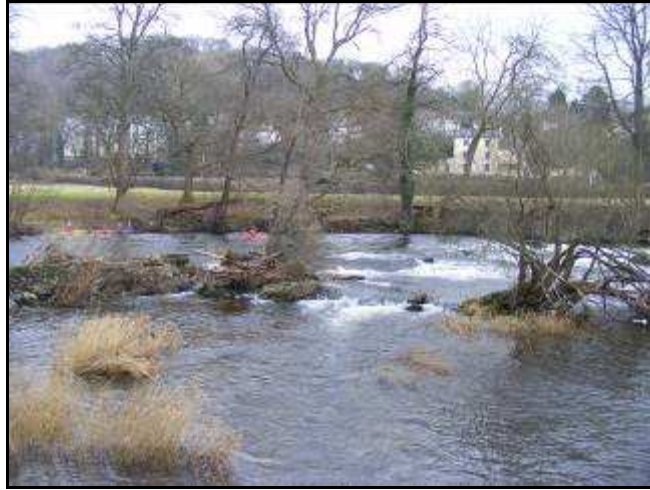
Figure 38 – Disrupted part of weir.
