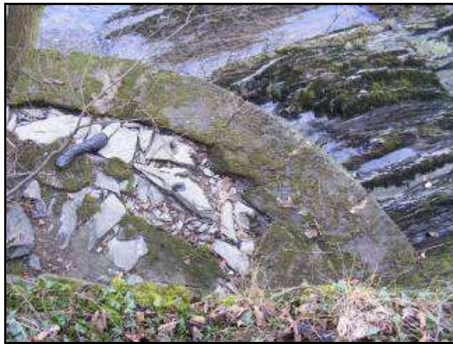
Figure 39 – Curved masonry structure in western bank adjoining western end of weir. Leat intake would have been immediately to the left of this.
