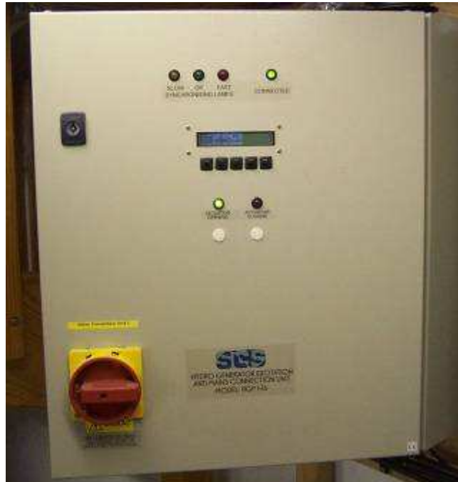
Figure 4 - Mains connection unit / hydropower system controller.
