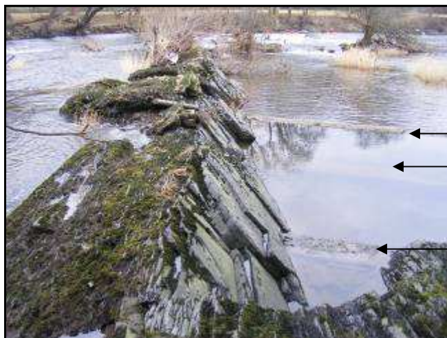
Figure 40 – Historic fish pass? Three masonry walls step down in height below the weir at its western edge.
