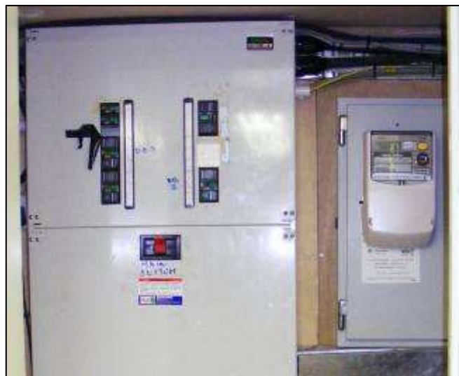
Figure 19 – Corn Mill electrical installation, showing three-phase main meter (top right) and main distribution board with spare ways (top left).
